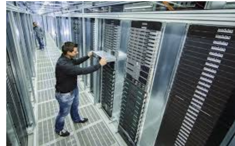
Many racks full of rack-mountable servers (data center)
